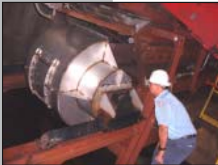
Teddy Scales, a Utilities employee, inspects the new "reclaim chute," designed by Jason Hollers. It recovers coal, reduces spill, and keeps belts moving smoothly after deliveries are made to the Central Heating Plant.
